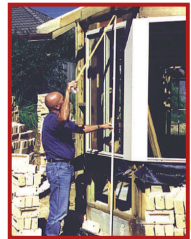
Measuring gauge to drop off point
